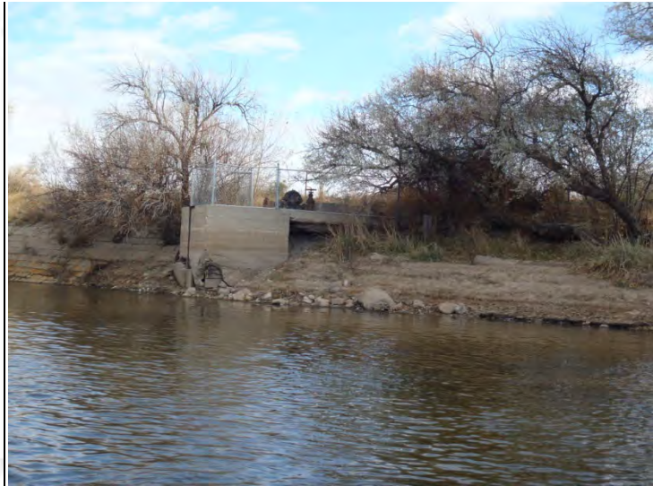
Concrete Pump Station Map-10-076
