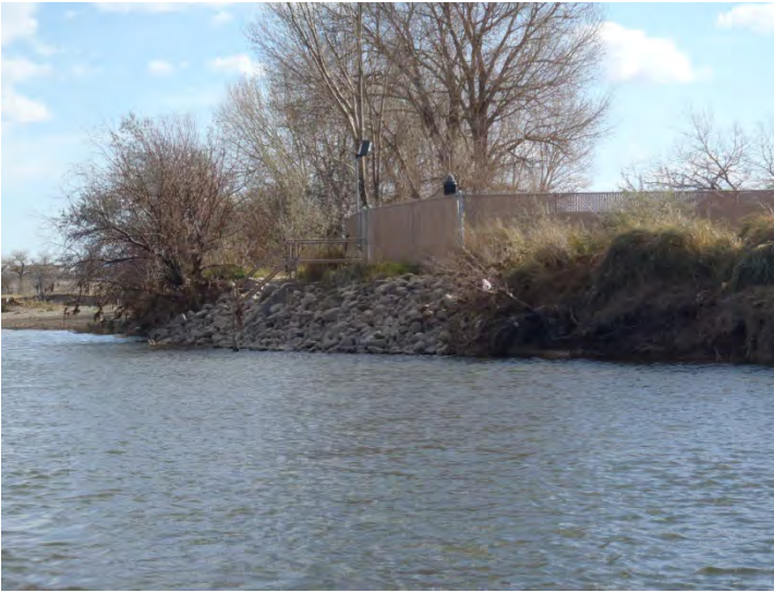
Pump Station Map-21-185
